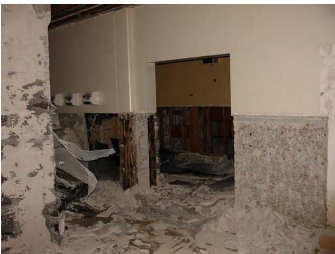
Hazardous Materials Abatement Required PE Complex, Volume II, Yuba College
