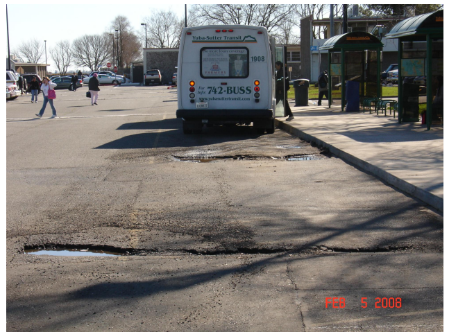
Bus stop pavement delamination. Repairs will be completed in February 2008.
