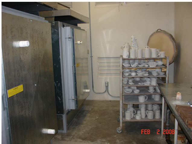
New gas-fired kilns in Room 1020, Building 1000.
