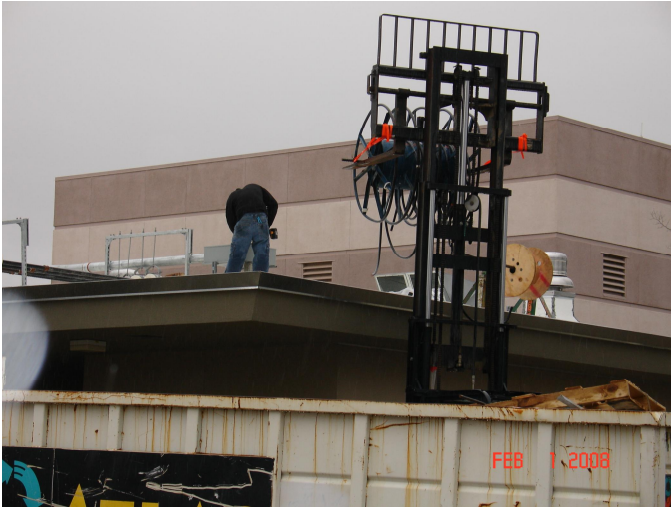
Electricians pulling power feeds into the South and West Wings for the Building 1000 renovation project.
