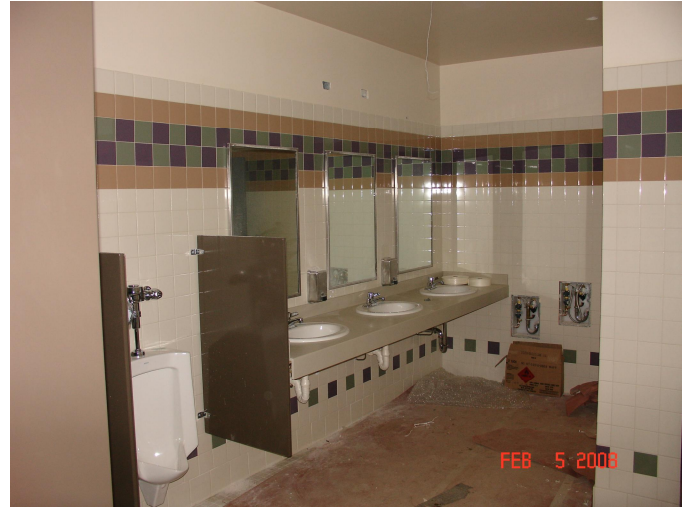
New bathroom in Building 1000. Just one aspect of the building's renovation project.
