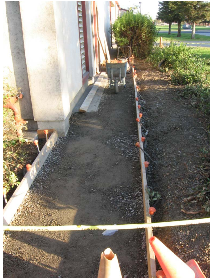
Exterior Improvements in conjunction with the Campus Police Relocation Woodland Community College
