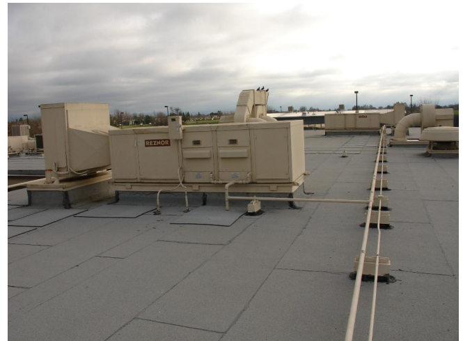
Make-Up Air Handling Unit to be Replaced Building 600, Yuba College
