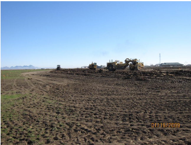
Developer Rough Grading of Future Project Site Colusa County Educational Outreach Facility
